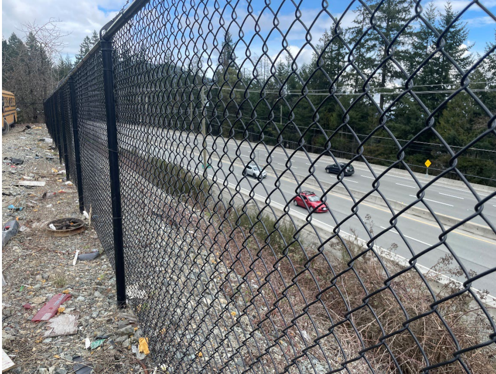
Photo 3: Typical chain link fence on east and south property line of 240 Okotoks Road.
