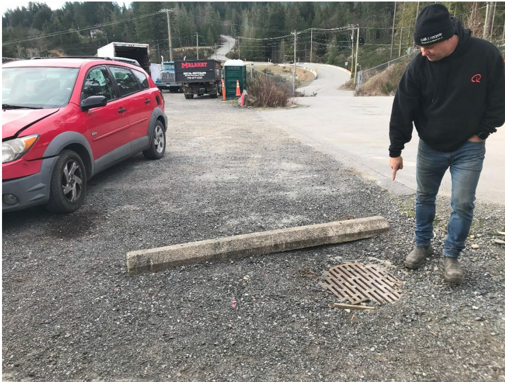
Photo 18: Slotted manhole cover in parking lot for overland flow and connected to the perimeter drain at 240 Okotoks Road.
