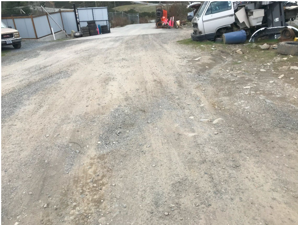
Photo 34: Depression flowing south to empty into the west ditch at the driveway entrance of 240 Okotoks Road.
