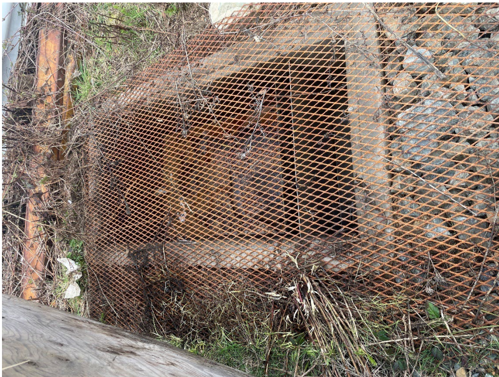
Photo 16: Rock pit connected to the floor drain in dome tent of the main office at 240 Okotoks Road.
