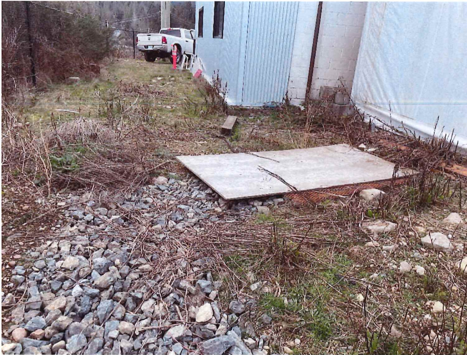
Photo 15: Location of rock pit connected to the floor drain in dome tent of the main office at 240 Okotoks Road.
