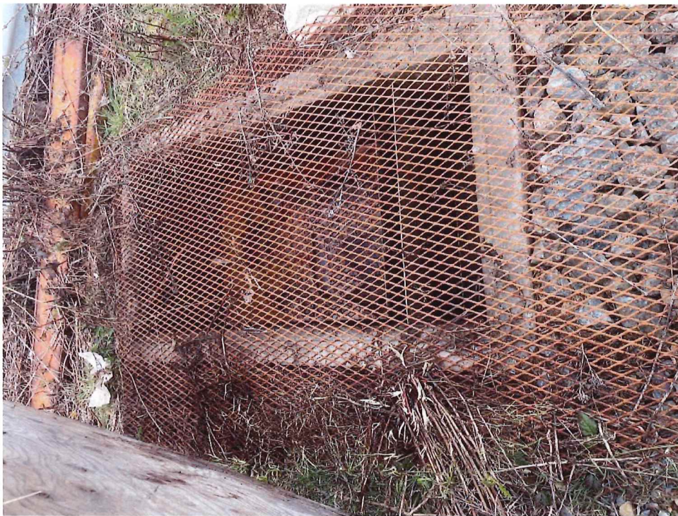
Photo 16: Rock pit connected to the floor drain in dome tent of the main office at 240 Okotoks Road.
