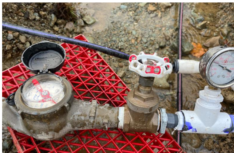
Figure 3 - Typical Flow Meter and Pressure Gauge
