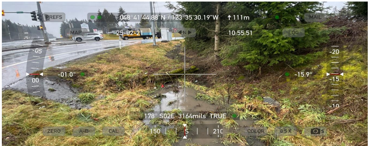
Culvert outfalls after cross draining under intersection to this Fisher Road ditch.
