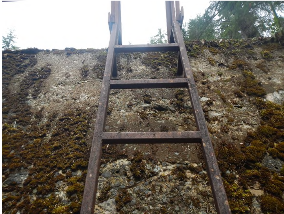
Photo 19 Weathering on the downstream face noted throughout the crest and front face.
