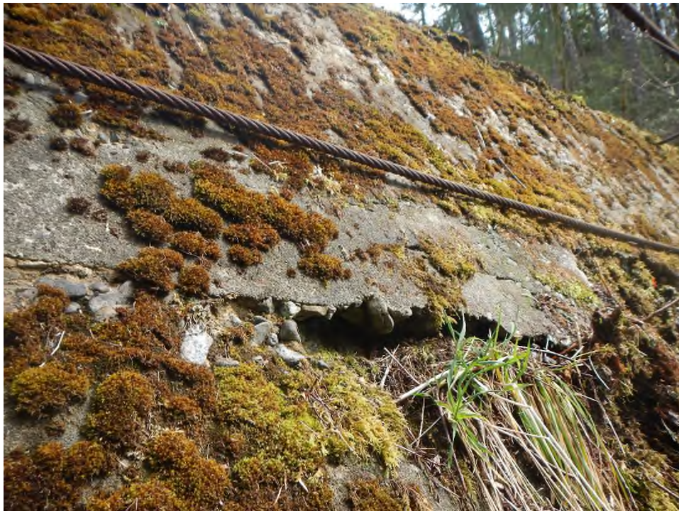
Photo 14 Horizontal cracking and erosion on downstream dam face approximately 1 m below the crest.
