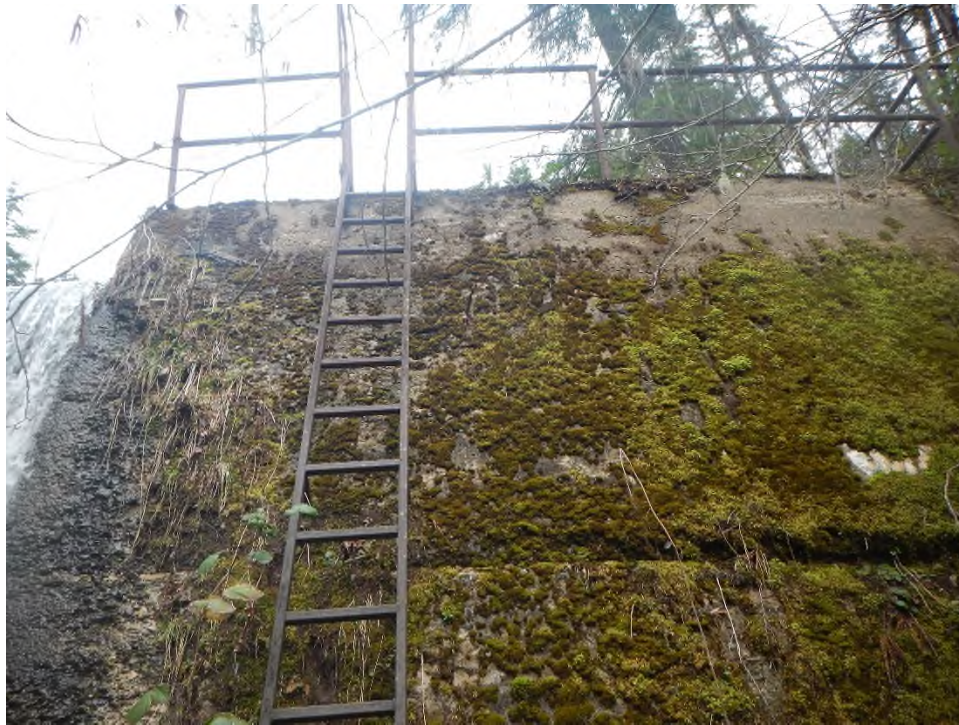
Photo 18 Horizontal groove on the left downstream face approximately 1.7 m below the crest.
