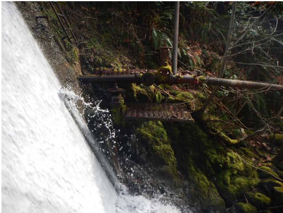
Photo 22 Low level outlet pipe and water intake line at left side of the dam.
