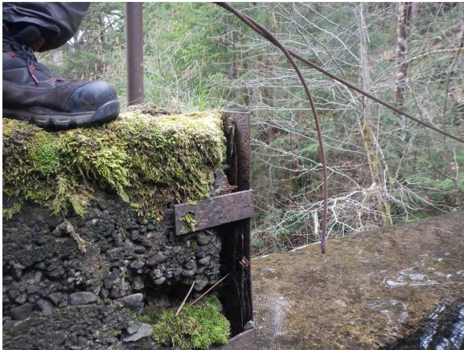
Photo 8 Weathering of concrete on the left side of the spillway at the stoplog insert.
