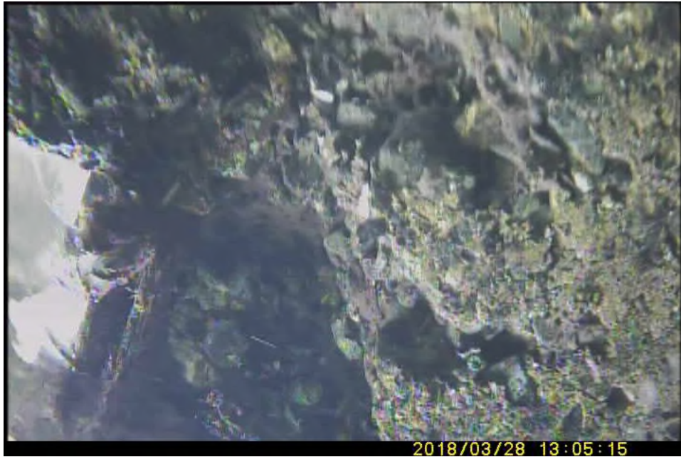
Photo 9 Concrete deterioration at edge of spillway.
