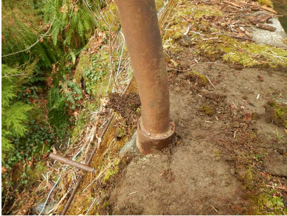
Photo 7 Corroded bent guardrail on the dam crest.
