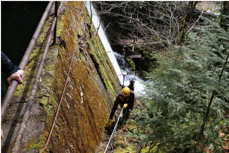
Photo 12 Downstream face of the dam as viewed from above at the right abutment.
