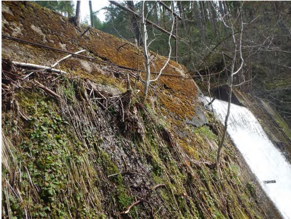
Photo 15 Vegetation growing on the dam face to the right of the spillway.
