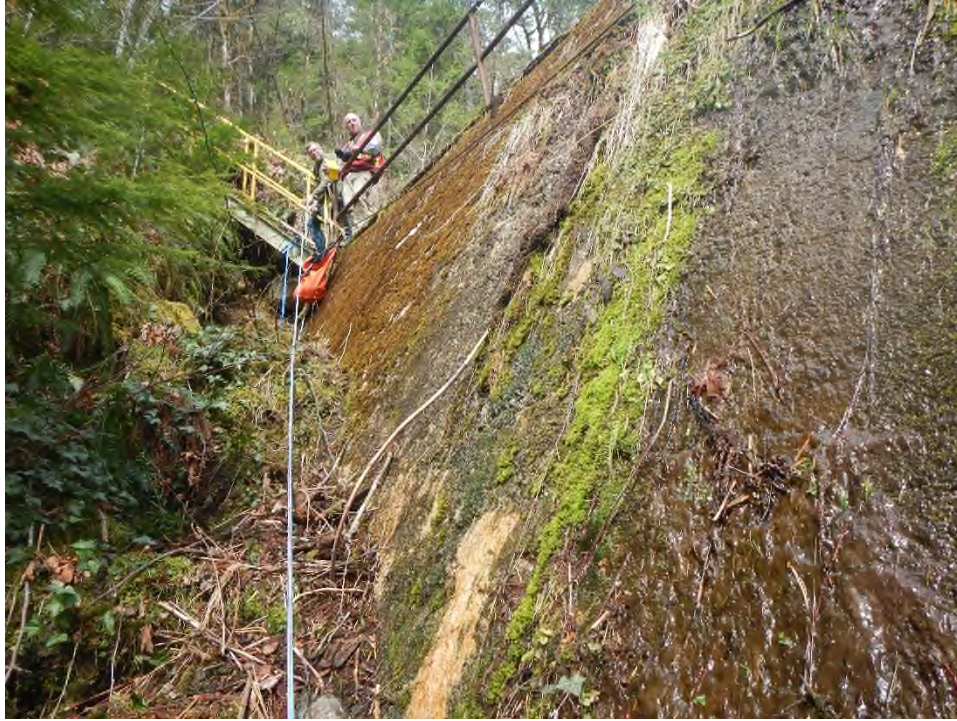
Photo 13 Downstream face of the dam as viewed from below looking towards right abutment.
