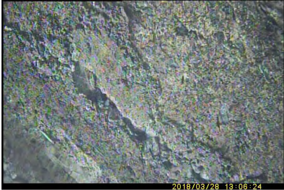
Photo 11 Backside of cold joint as viewed from within the reservoir.
