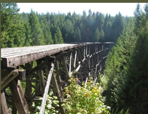
Kinsol Trestle before rehabilitation
