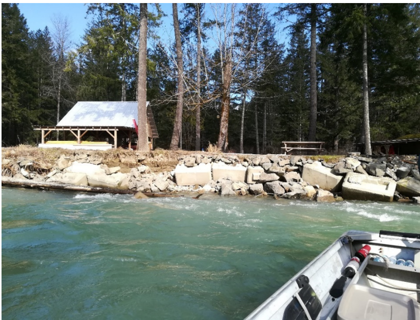
Photo 3: Example of damage to bank protection works along private property, 18 February 2020
