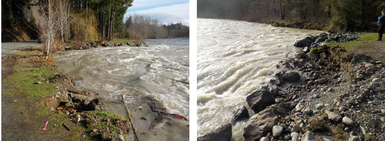
Photo 4: Severe overtopping and scour damage to riprap revetment along Riverbottom Road near Jenny Place, 1 February 2020
