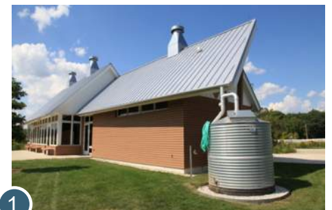
Above Ground Rainwater Harvesting System ( www.completeenergyuk.co.uk )
