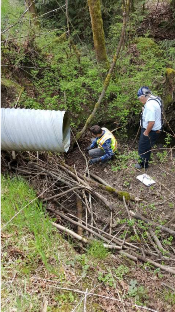
Photo 4: Inlet of Tzingua Road Twin Culvert (lower culvert blocked)
