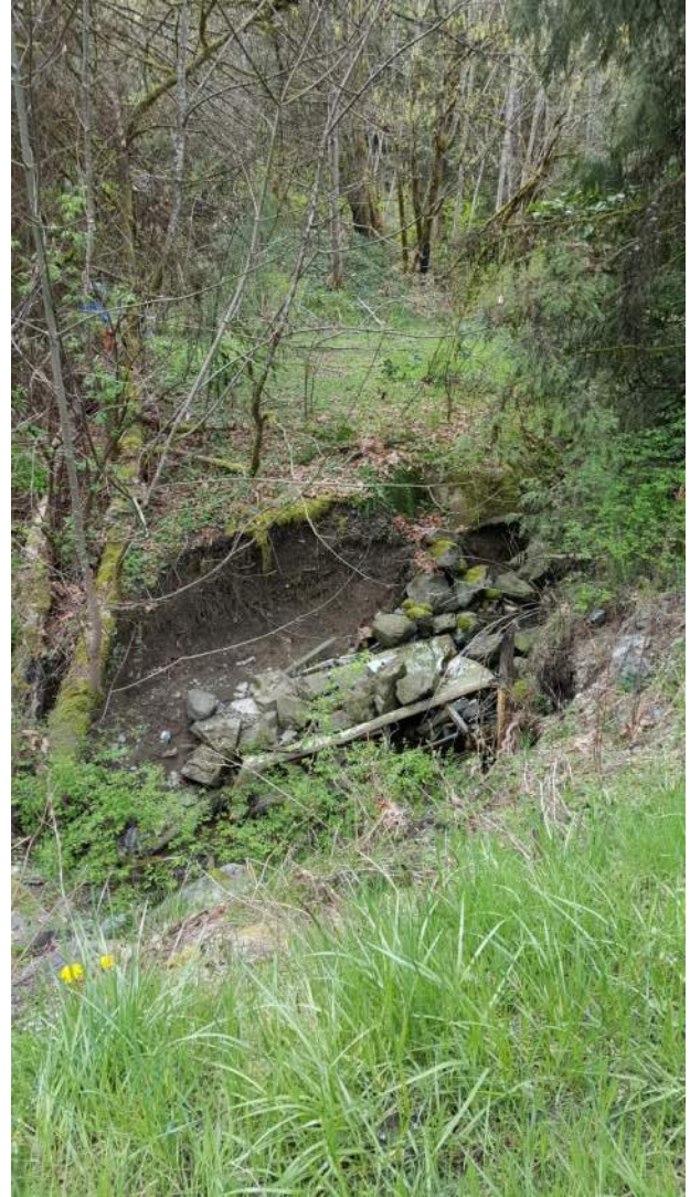
Photo 5: Bank Erosion at Miller/Koksilah Road Culvert Crossing (upstream side)
