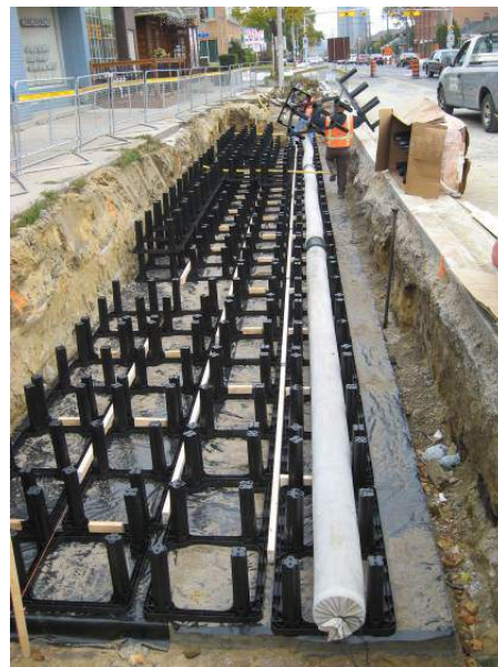
Perforated drain line is installed at the bottom of the 1st layer of Silva Cells and connected to the catch basin.
