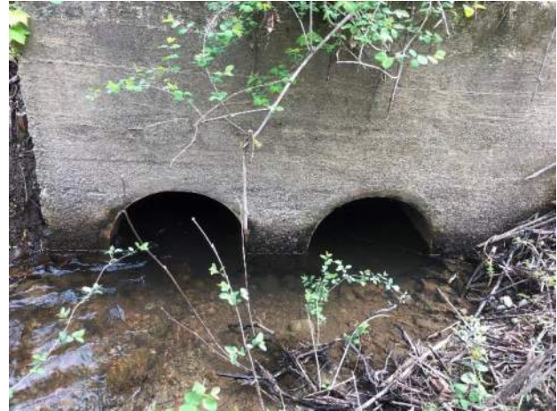
Twin 450 mm diameter culverts under E&N Railway
