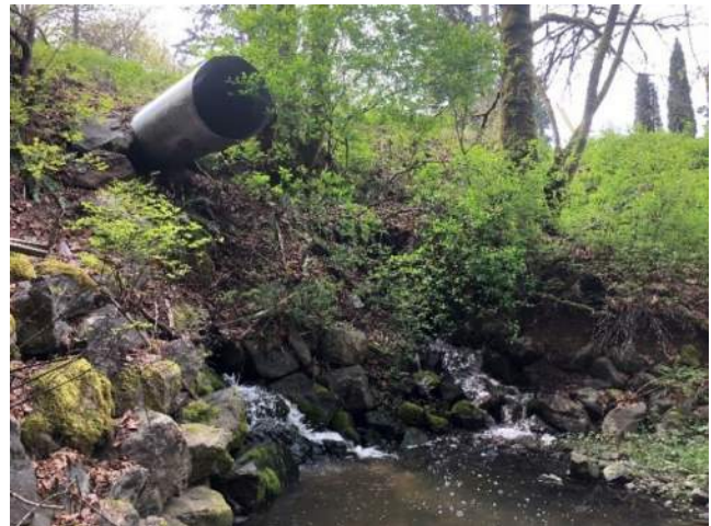
Koksilah Road/Miller Road Culvert Crossing showing complete obstruction of fish passage.
