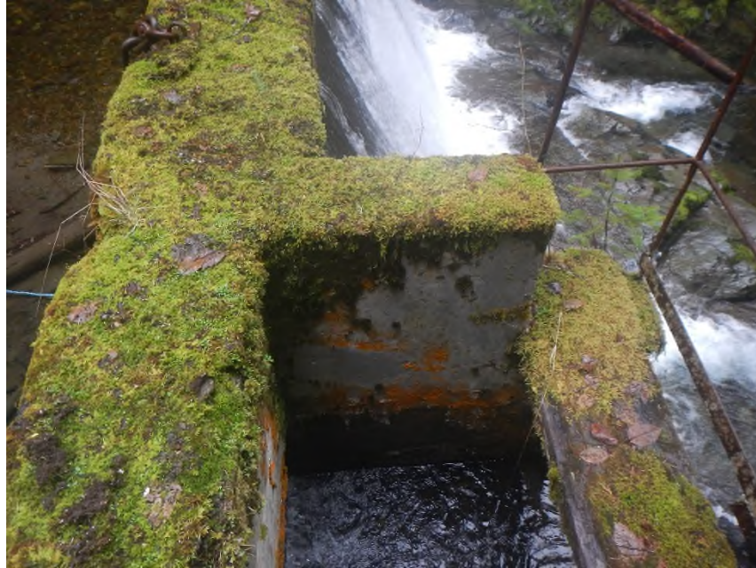
Photo 11 Moss growing on dam reducing visibility.
