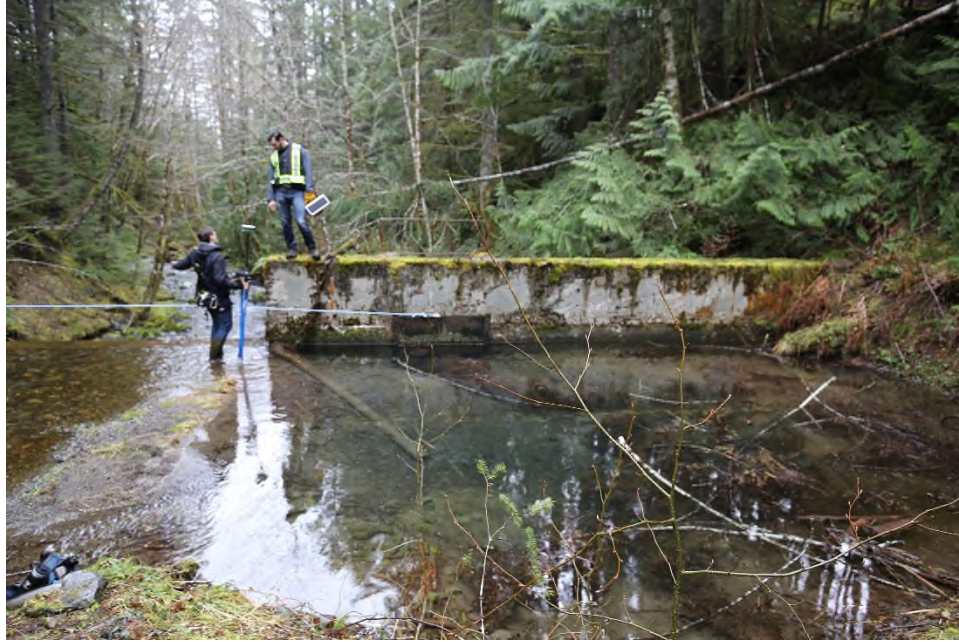
Photo 3 Right wingwall viewed from upstream. Erosion and weathering noted.
