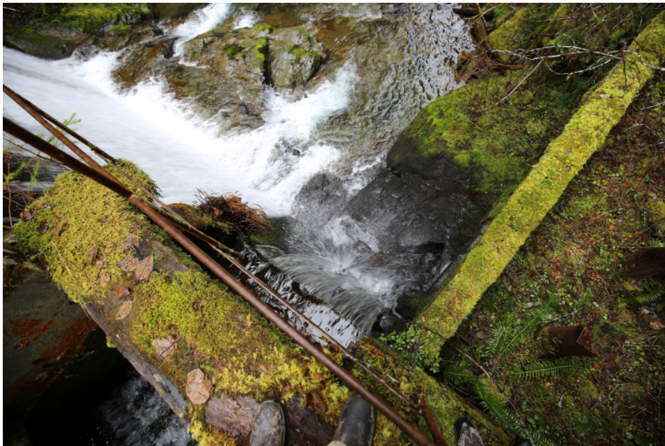
Photo 8 Downstream wingwall and area of downstream discharge of smaller channel.
