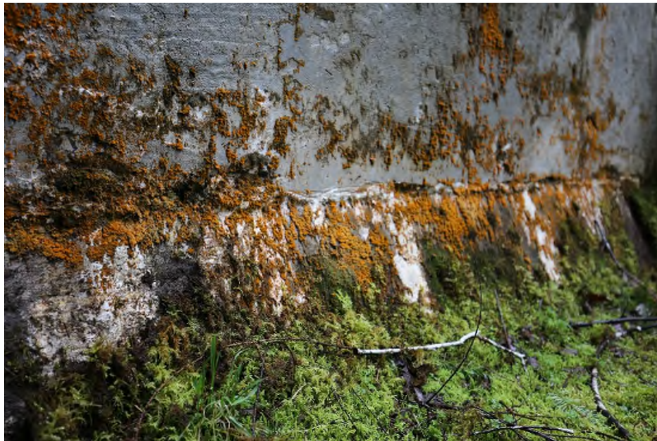
Photo 14 Cold joint at the right side of the dam between headwall and sloped part of the structure. Looking towards spillway.
