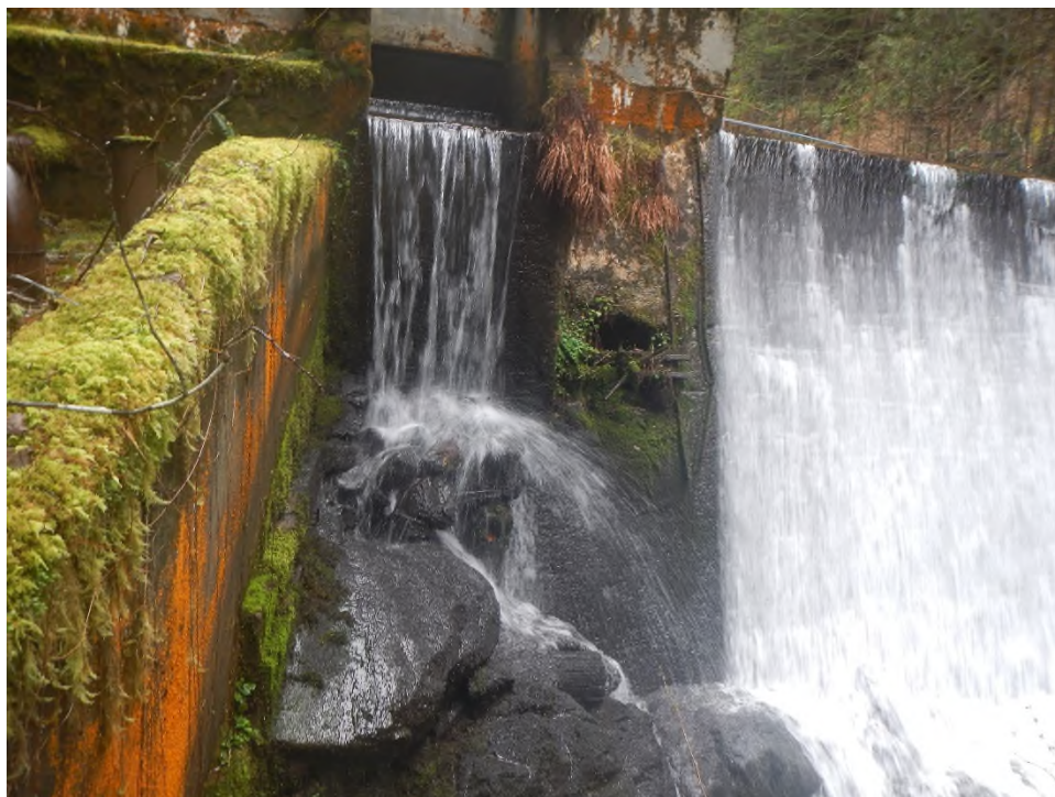
Photo 17 Spillway channels viewed from wingwall. Outlet in center is blocked.
