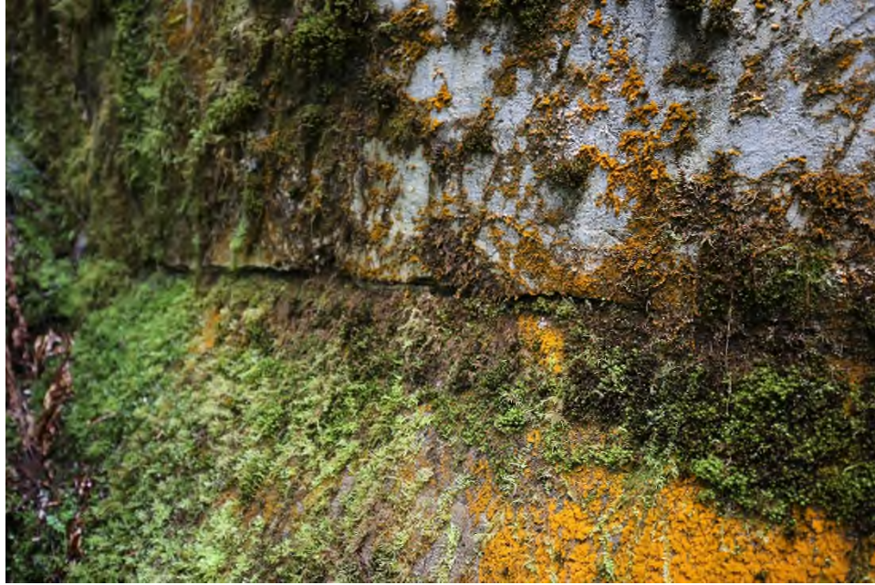
Photo 13 Cold joint at the right side of the dam between headwall and sloped part of the structure. Looking towards abutment.
