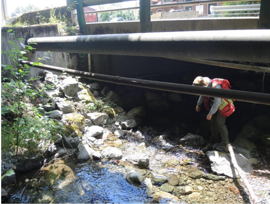
Figure 16. The Highway 18 bridge crossing over Coonskin Creek. It may be capable of passing small debris flows and debris foods. Exposed utilities on the upstream side of the bridge are vulnerable to impact from transported debris.
