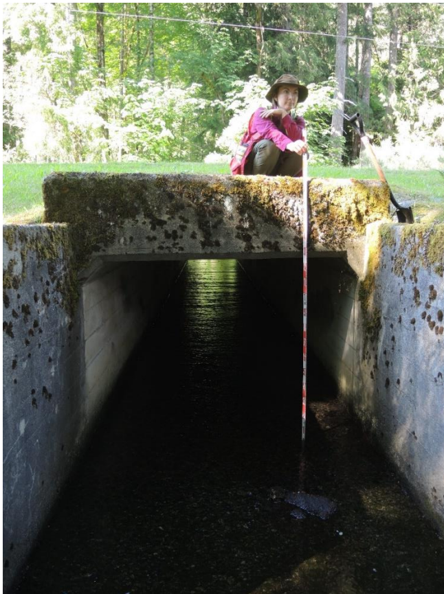
Figure 15. The 1.2 m high x 2 m wide, concrete box culvert on the Swordfern Creek crossing. This structure is unlikely to pass debris from debris flows or debris floods.
