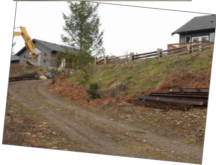
Rear of House Showing Slope, Dismantled Building Parts & Start of Drainage Works
