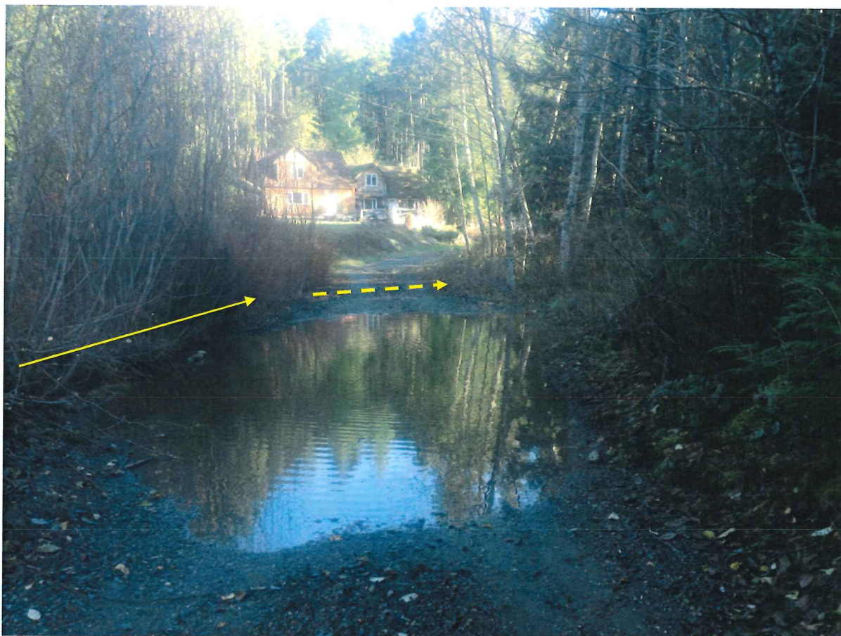
Figure 12. Looking east along the driveway that parallels the north property boundary. The dashed yellow arrow is the approximate location of the blocked culvert under the driveway. The solid yellow arrow is the alignment of a stream/pond that flows across the driveway, given the blocked culvert. Photo taken November 21, 2016.
