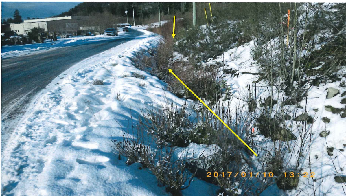
Figure 14. Looking west toward the cul-de-sac at the end of Ark Road. The solid yellow arrow is the location of the culvert crossing under Ark Road. The yellow arrow shows the direction of runoff flows. Photo taken January 10, 2017.
