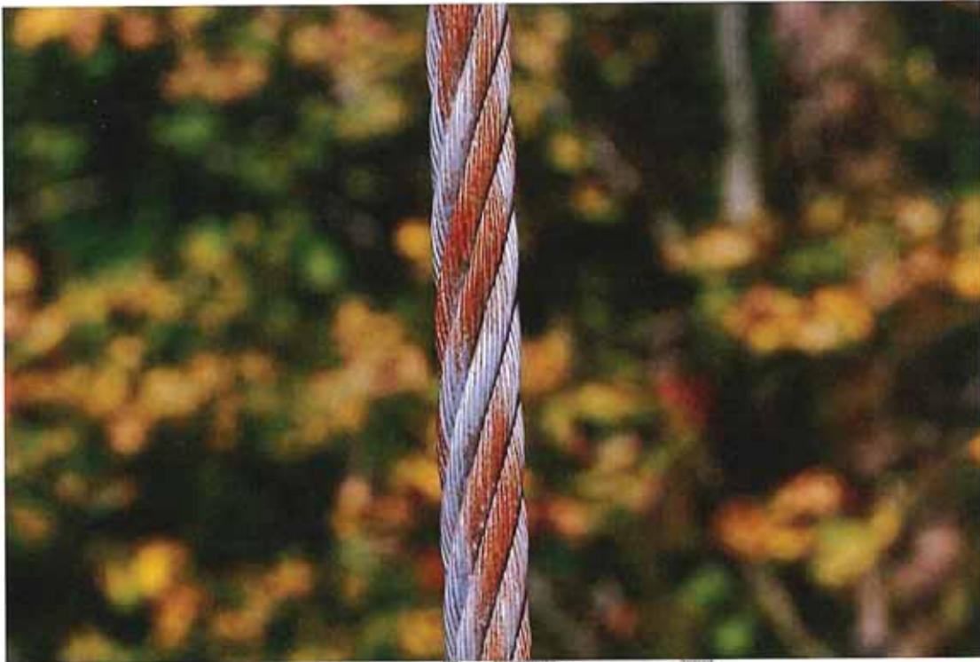
Figure 11: Surface Corrosion on Hanger Cable
