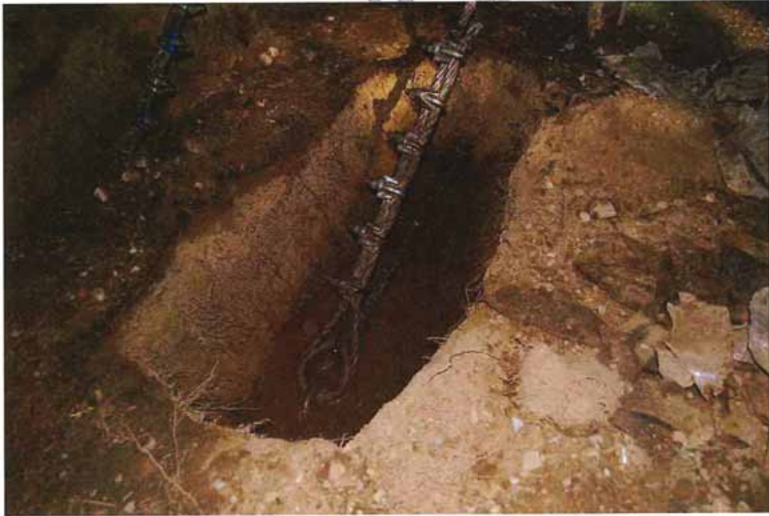
Figure 6: Unwrapped Cables at West Anchor
