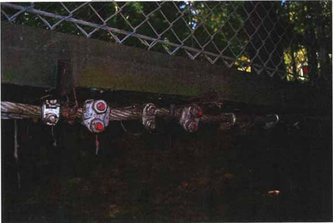
Figure 8: Walkway Cable Splice
