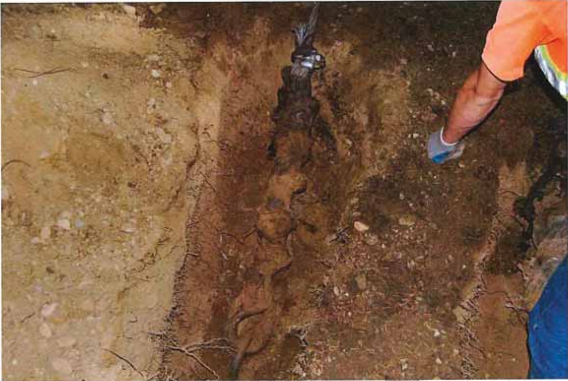
Figure 5: Wrapped Cable at West Anchor
