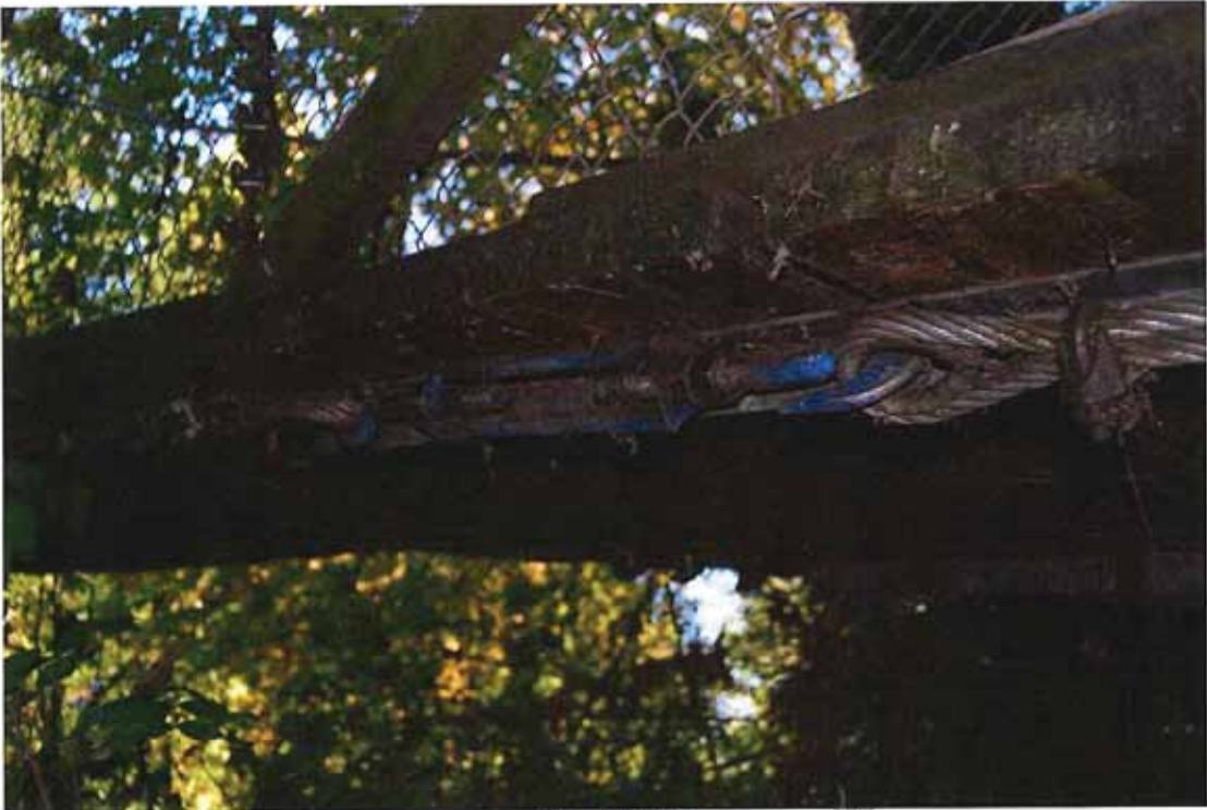
Figure 7: Walkway Cable Turnbuckles
