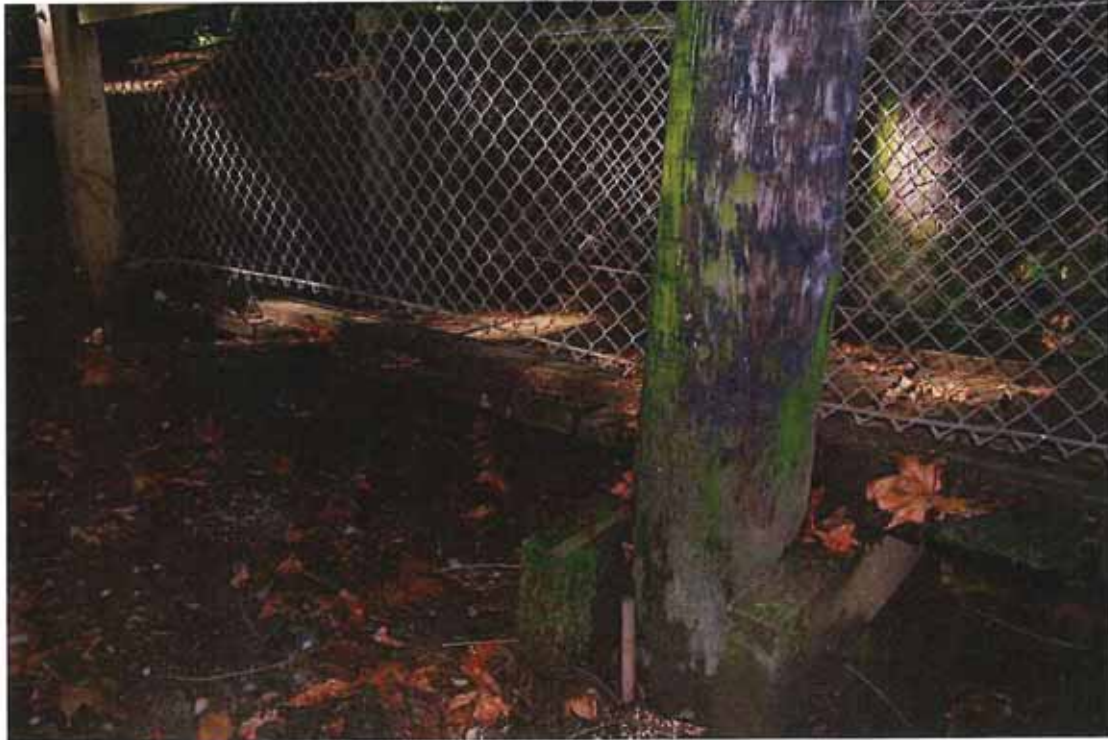
Figure 14: Tower Post Base with Decay
