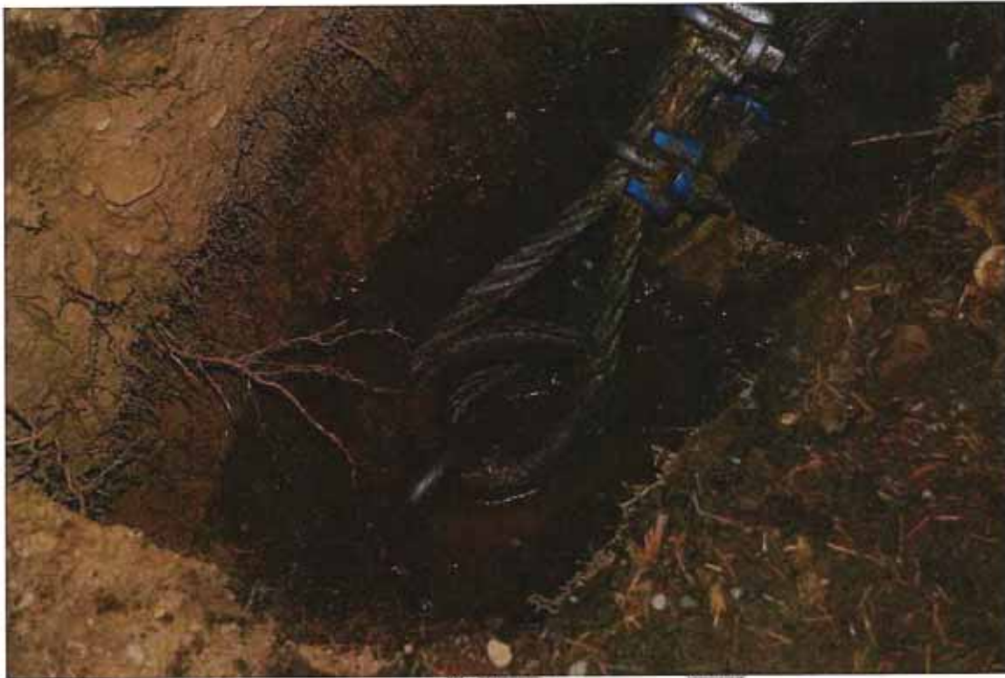
Figure 15: Improperly Clipped Turn-Back Eye with Rotated Thimble
