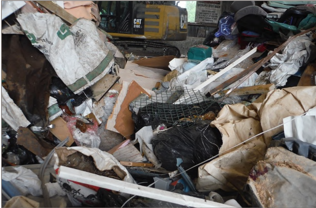
Photo 13: C&D – Durable plastics, other building material, drywall/gypsum, contaminated wood, among others identified.
