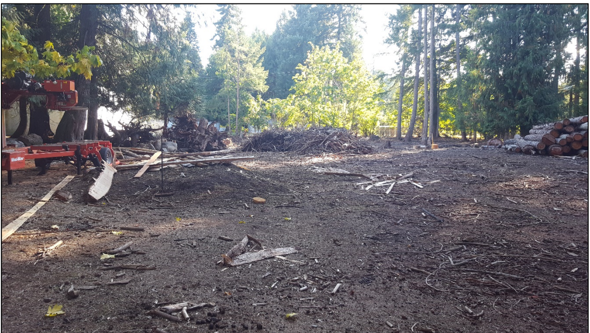
Photo 4. Showing the cleared area adjacent to the fire station where the new building is planned to be constructed. Facing south towards Yellow Point Road with the existing fire station visible on the left side of the photo.
