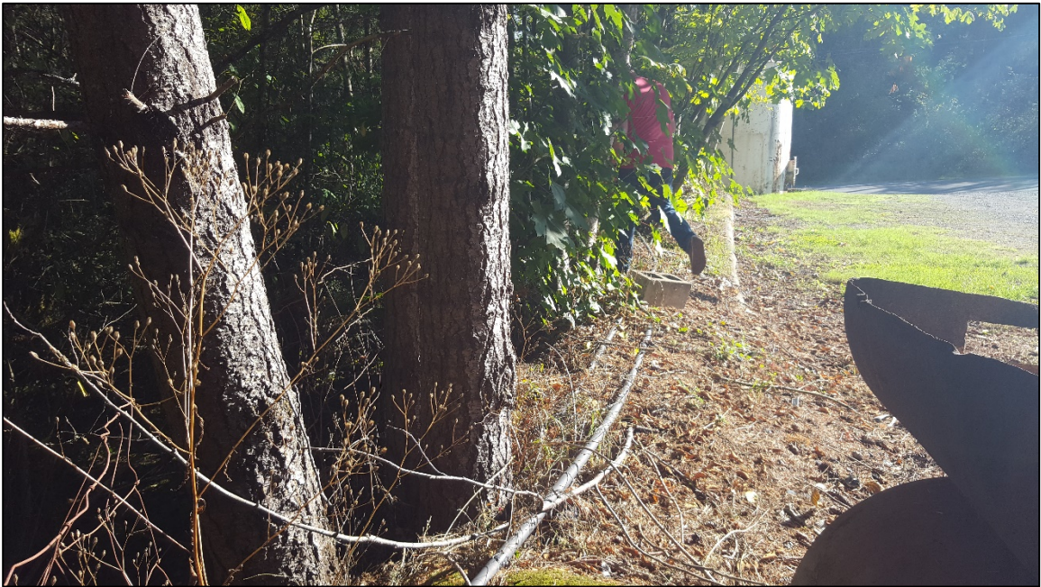
Photo 3. Showing the concrete retaining wall on the eastern edge of the parking area. The wall is partially buried and the trees in the foreground would require removal for retaining wall replacement.
