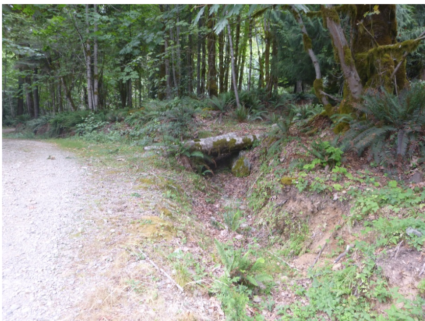
Photo 10. The ditch network (Ditch 3) adjacent to the access road for proposed Lot D. Note the vegetation growth, which is an indication water has not flowed through the ditch in a prolonged period of time.
