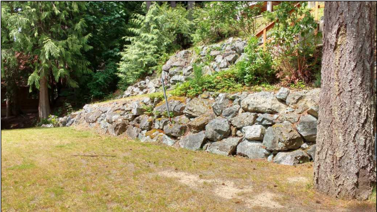
Photo 14 – Looking northwest at the third and fourth riprap retaining walls up from the lake, taken from the second terrace at the east property boundary.
