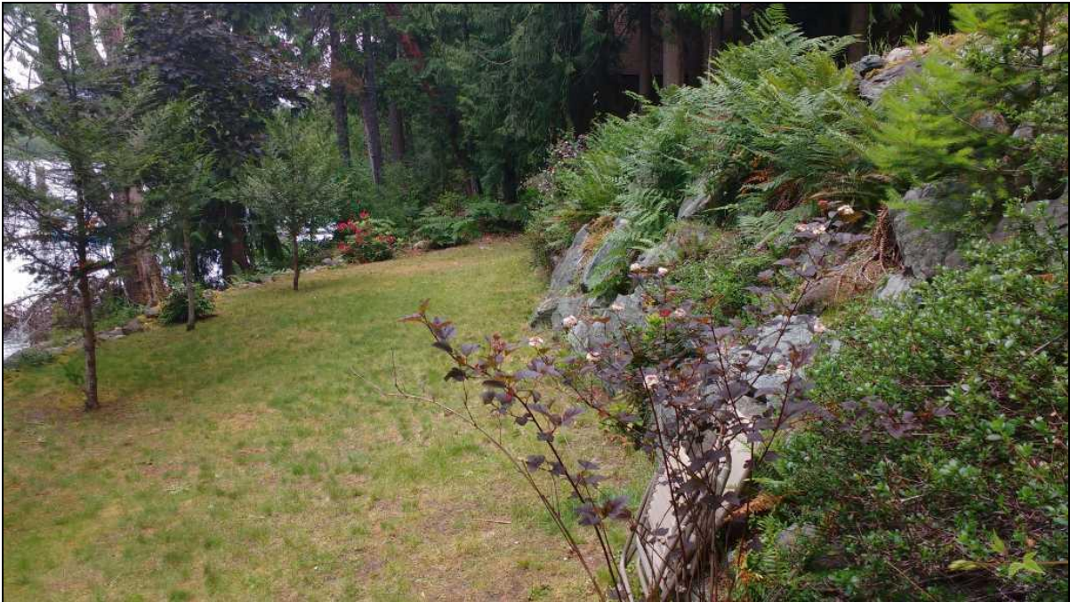
Photo 16 – Looking west along the first terrace and second riprap retaining wall up from the lake.
