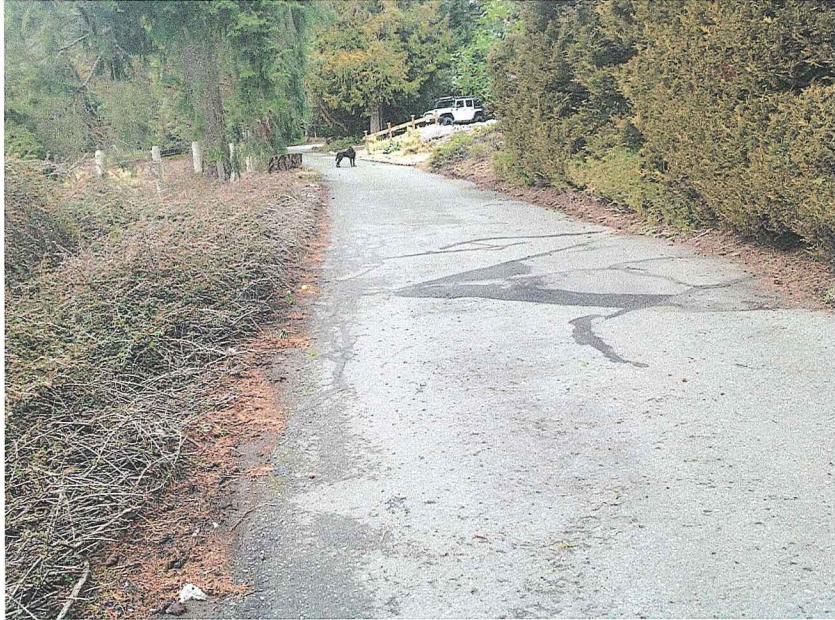
FRONT PAVED DRIVEWAY FACING WEST
