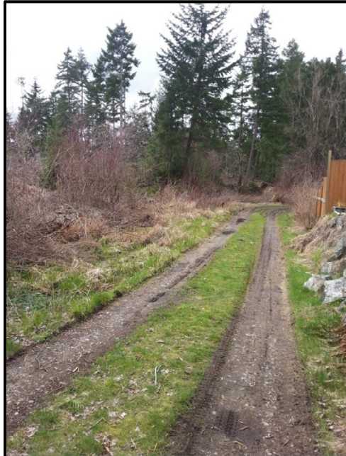
Looking west along the existing service road, which borders the northern boundary of the property. This road appears to flood during events containing high amounts of precipitation.
