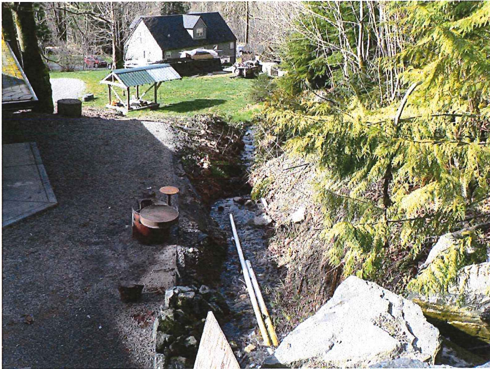
Photograph 7. View downstream from pipe outlet with eave overhang and patio visible on left.
