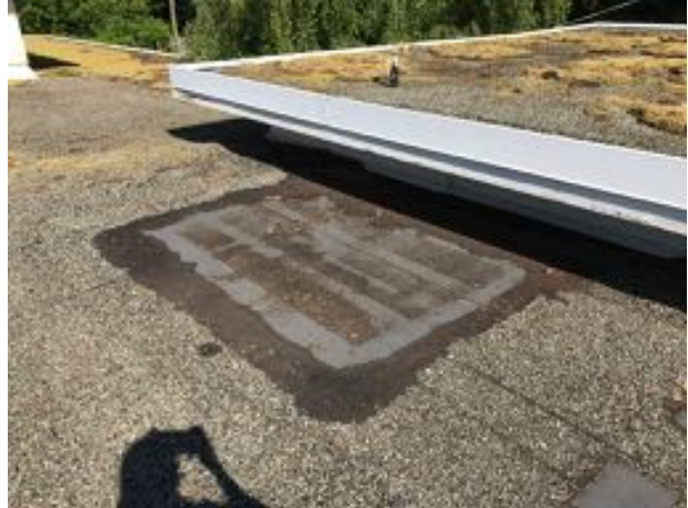
Photo 10 – An evidence of past repair
