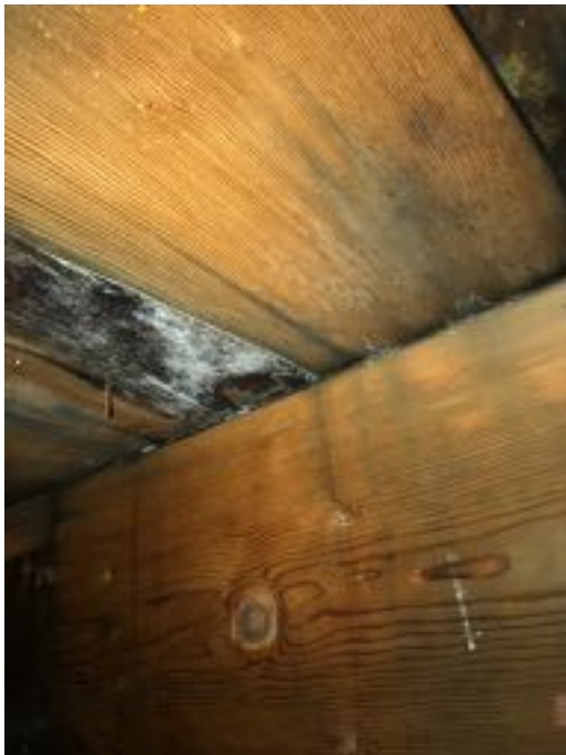
Photo 15 – Rusted nail penetrating through sheathing above and stains and microbial growth on wood members
