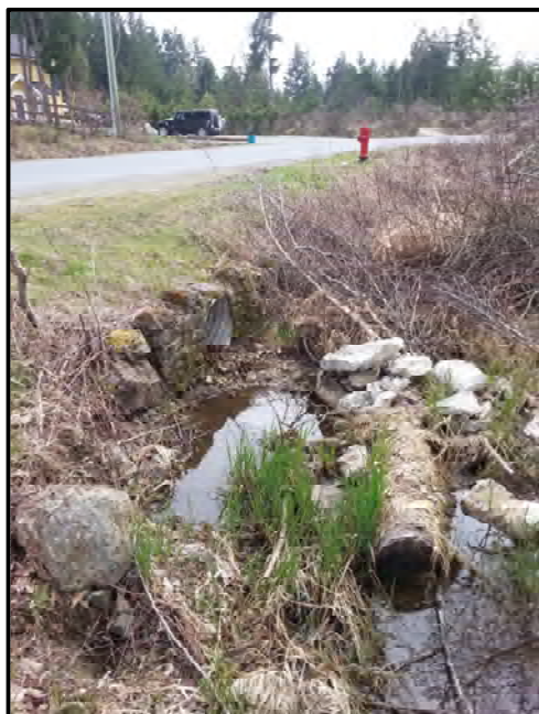
A representative photo of the outlet of the CMP that directs stormwater runoff onto the subject property.
