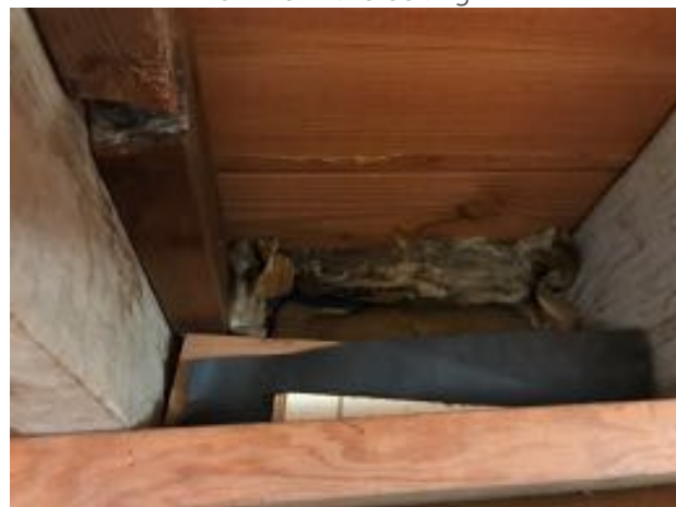
Photo 19 – Water stains and microbial growth on wood members
