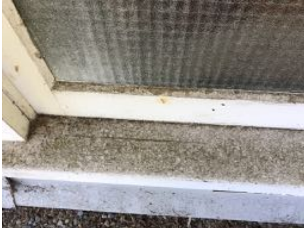
Photo 29 – Microbial growth and deteriorating paint finishes at window frame and sill
