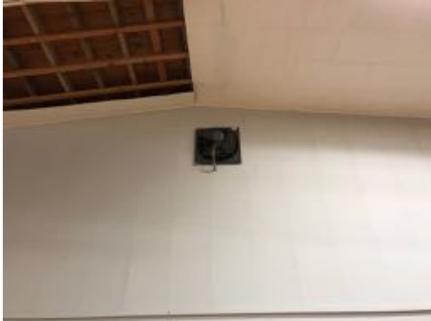
Photo 20 – Ghosting of studs on south wall and fan
