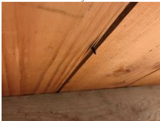
Photo 18 – A nail penetrating through the wood decking
