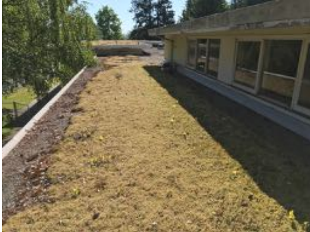
Photo 9 – Extensive moss covering the north side of the roof
