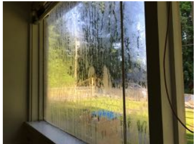
Photo 26 – Close up of the condensation on window glazing
