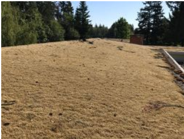
Photo 5 – Extensive moss covering the roofing
