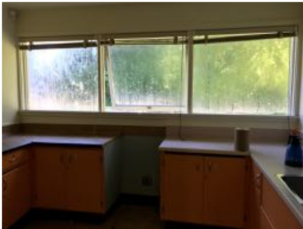
Photo 25 – Condensation and fogging on the inside face of glazing
