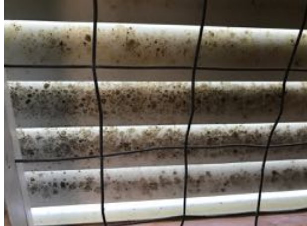
Photo 30 – Microbial growth on window covering
