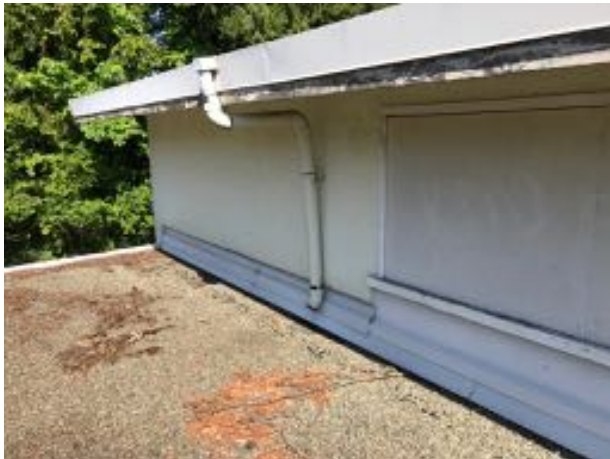
Photo 23 – Typical attachment of rain water leaders to the exterior wall without any sealant around the fasteners
