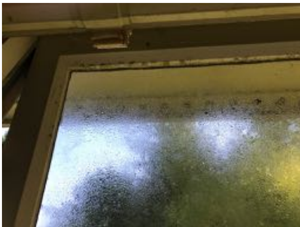
Photo 27 – Microbial growth around window around the glazing perimeter
