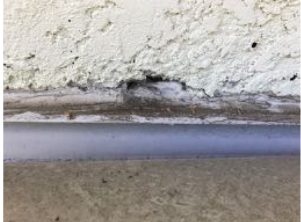
Photo 22 – An opening above the flashing and sealant due to uneven stucco at base of wall
