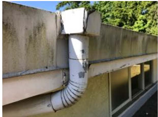
Photo 6 – View of a scupper and rainwater leader in poor shape
