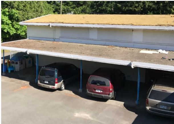
Photo 31 – Boarded up windows of on south elevation
