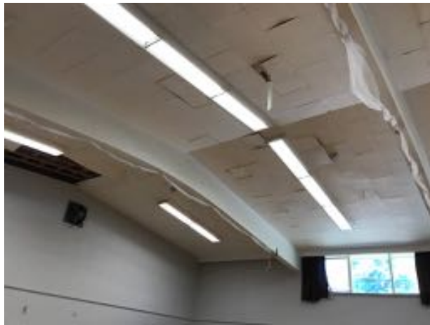
Photo 16 – Bulging and sagging ceiling tiles throughout
