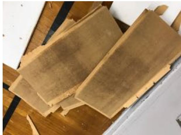
Photo 17 – Backside of the ceiling tiles that fell off from the ceiling
