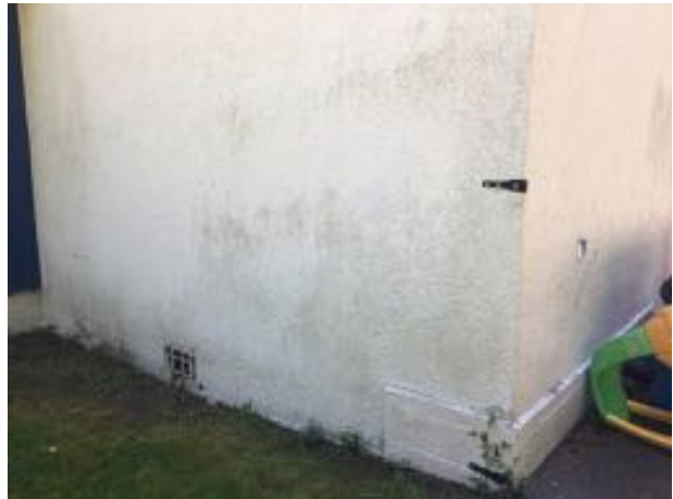
Photo 24 – View of north wall where stucco cladding terminates at grade
