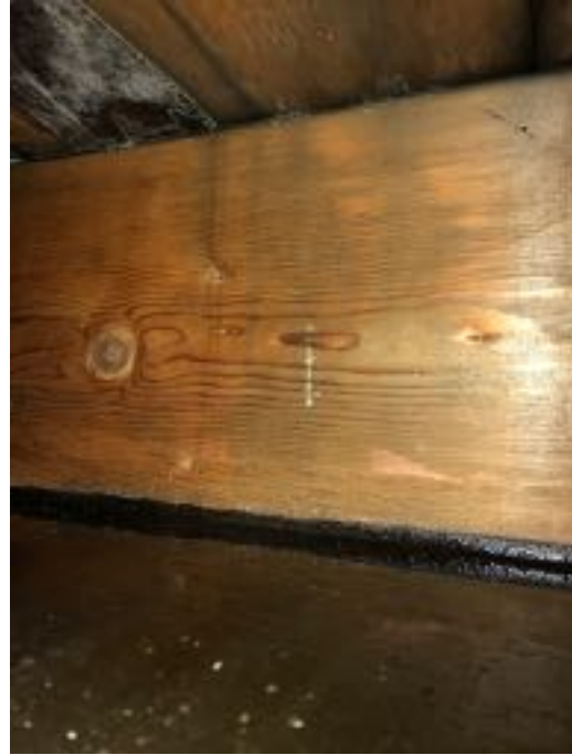
Photo 14 – Pooling water sitting on soffit
