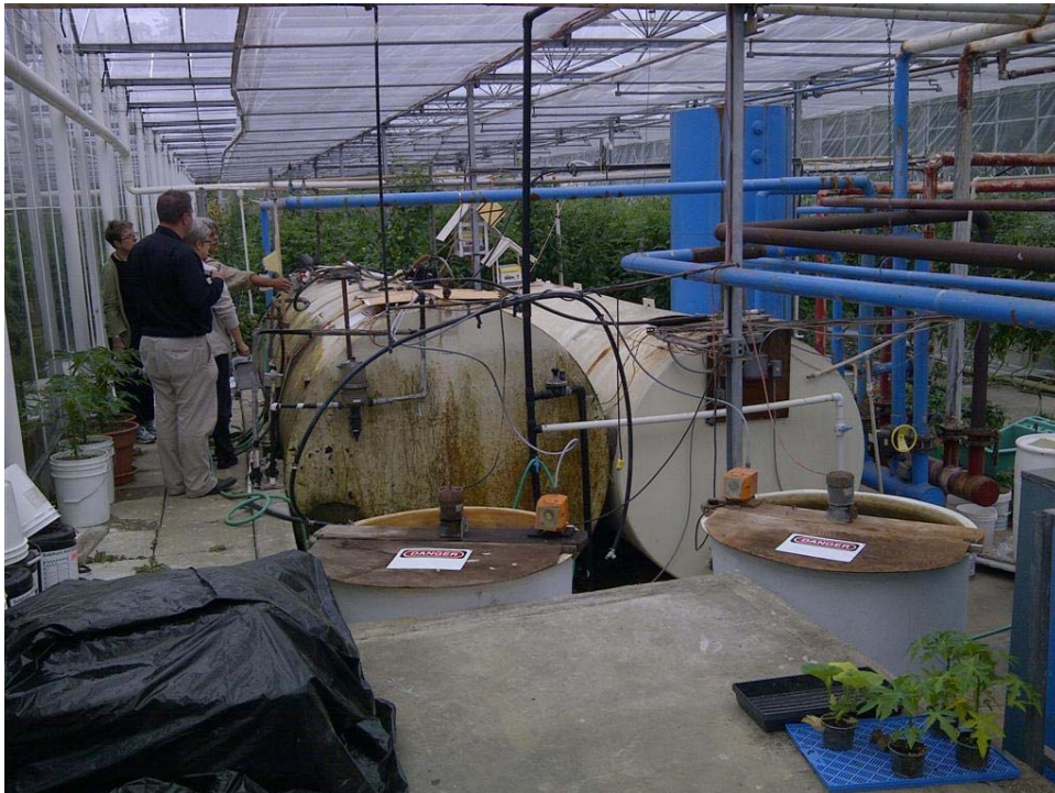
Photo 10: Irrigation water holding tanks and mixing area at 1360 Fisher Road.
