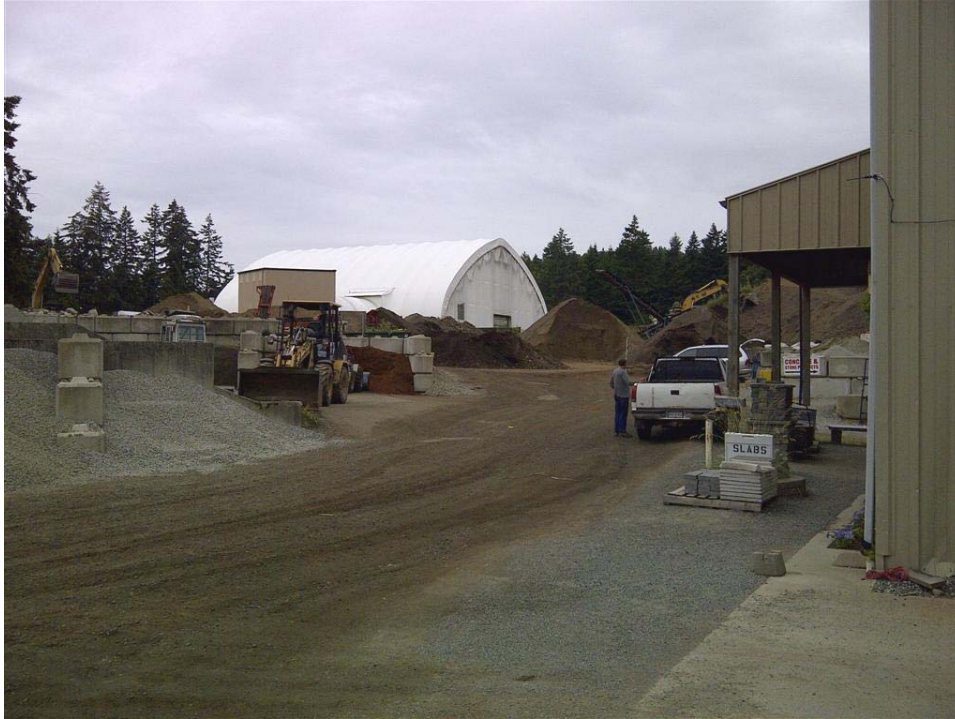
Photo 11: Looking west towards the stockpile holding and processing area at the central and west side of 1345 Fisher Road. The large white building in the distance is the compost receiving building at 1355 Fisher Road.
