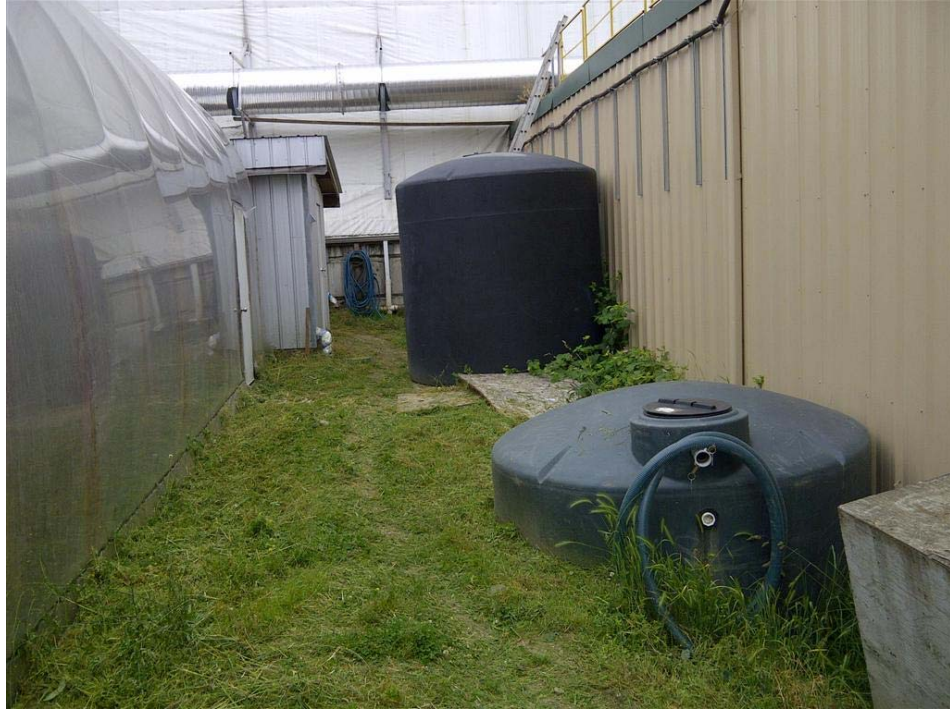
Photo 5: Looking north towards the compost curing (receiving) building with the composting vessels building on the right and bio-filter building on the left. The green tanks are used for temporarily holding any excess leachate generated in the vessels. The small shed (background left) holds a tank used to temporarily store and treat collected condensation water.
