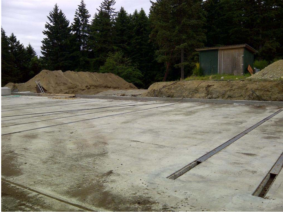
Photo 3: Looking west at the existing well shed (on right) with an air floor curing pad in the foreground.
