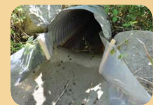
Directive fencing to encourage toadlets to cross under the road through an existing culvert.
