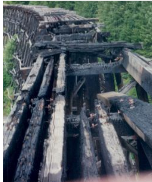
The damage to the trestle after the fire
