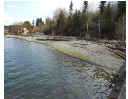
View of the Green shores work looking southeast from the new Cowichan Bay Marine Gateway site
