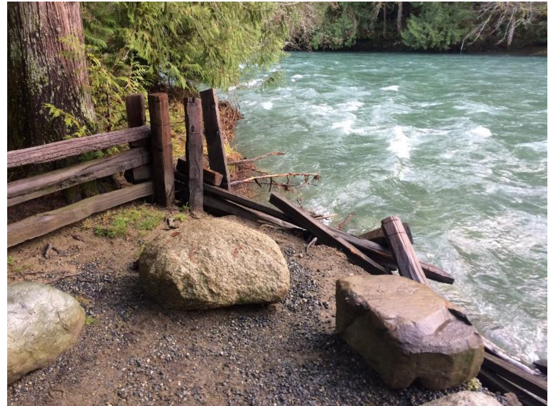
Erosion damage to park infrastructure and increased public risk exposure
