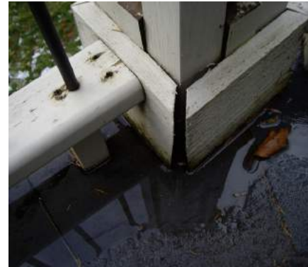
Top mounted guard posts should be avoided
