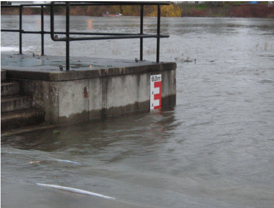
Photo 2: Highwater mark on outlet of Beverly Street pump station, Nov 20, 2009.
