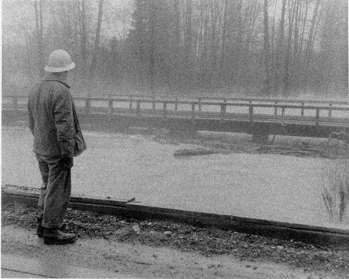
Log jam forming at upstream end of bridge.
